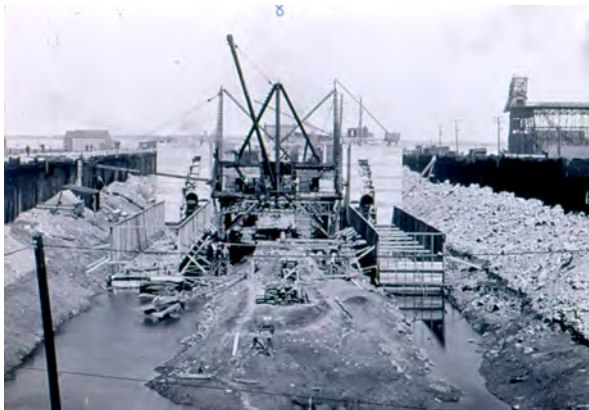
Black Rock Lock under construction, circa 1912. Photo courtesy historical archives of the US Army Corps of Engineers.
